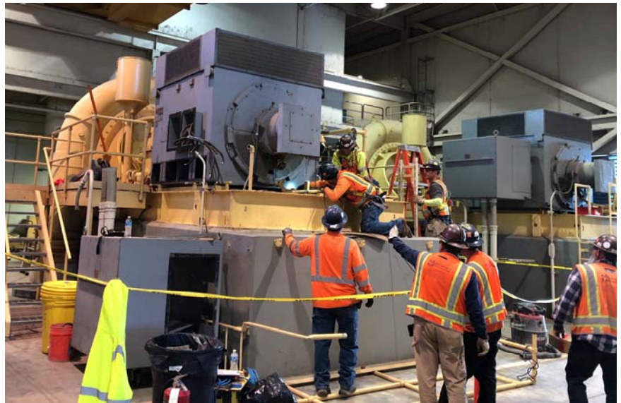
Figure 1: Contractor prepares to remove blower motor as part of the Blower Rehabilitation Project
