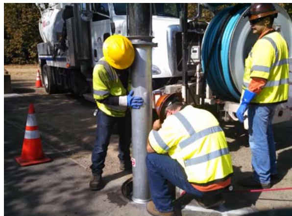
Clean-Out of a Continuous Deflective Separation unit installed in the Selma Olinder neighborhood
