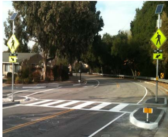
Flashing Beacons on Coyote Road & Crosslees Drive
