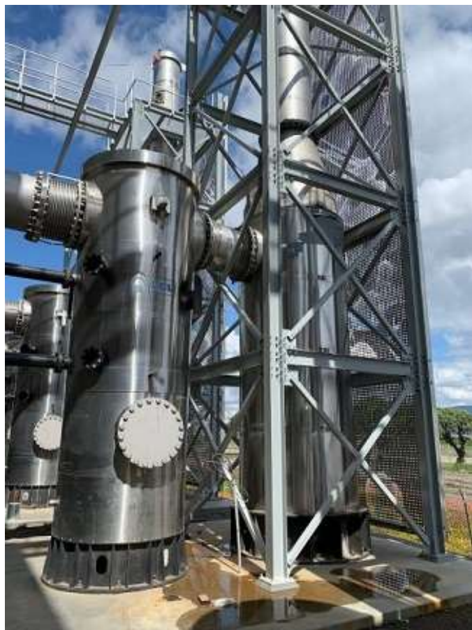
Figure 8: The new engine generators' high exhaust heat is used to produce hot water, which is then used to provide heat to the digesters and other facilities. The exhaust gas is cleaned through a treatment system before being discharged through the exhaust stacks.
