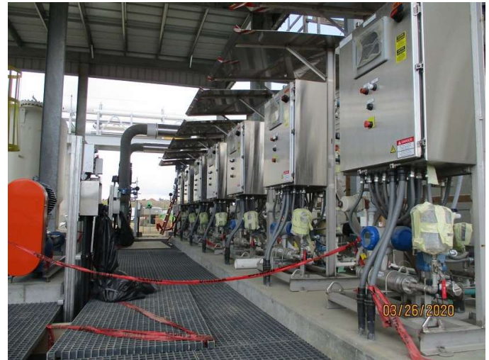
Figure 10: The automated polymer blending system will feed polymer to the blended sludge prior to entering the dissolved air flotation thickener tanks.
