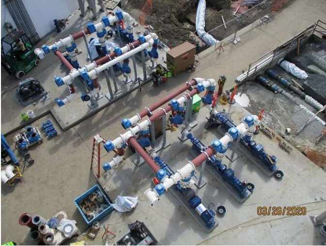
Figure 9: The upgraded foam suppression and withdrawal pumps and visible piping for thermophilic Digesters 5 and 7.
