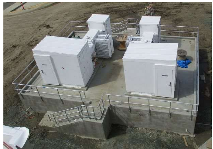
Figure 12: The new electricity load center at 5th and Center Streets will reduce the grid voltage to power the digester equipment.
