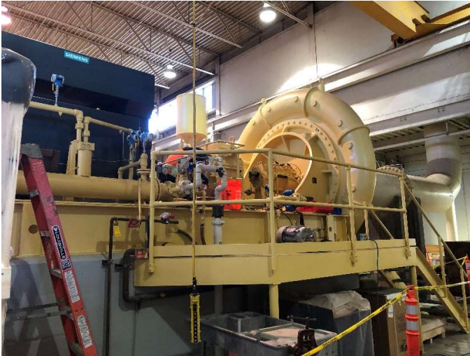
Figure 2: Reoriented and refurbished mechanical system, including a new motor and various utilities connections, for one of the blowers in the Power and Air Building.
