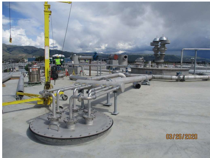
Figure 11: The Digester 5 gas withdrawal system is comprised of injection piping shown nearest, and pressure relief valves and digester gas separators in the distance. The digester gas will be used by the new Cogeneration Facility engines to generate electricity and heat for the RWF.
