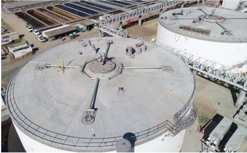
Figure 1: Aerial view of the Digester 5 (left) and Digester 6 (right) gas withdrawal system
