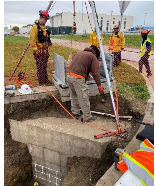
Figure 3: The contractor prepares the existing electrical conduit system maintenance access point for additional conduit connections. The existing rebar locations are marked on the outside of the concrete junction structure to guide new conduit positioning.
