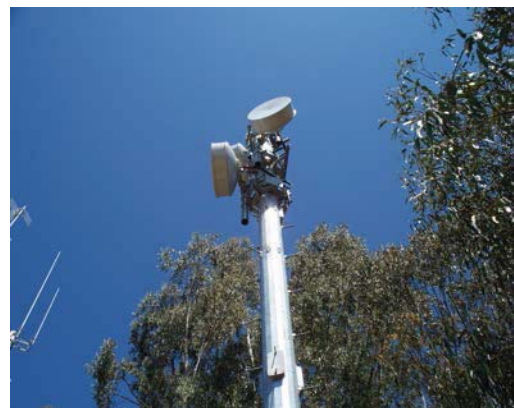
ECOMM Antennae at Eagle Rock
