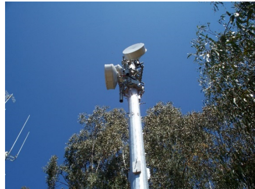
Emergency Communications Microwave Antennae at Eagle Rock
