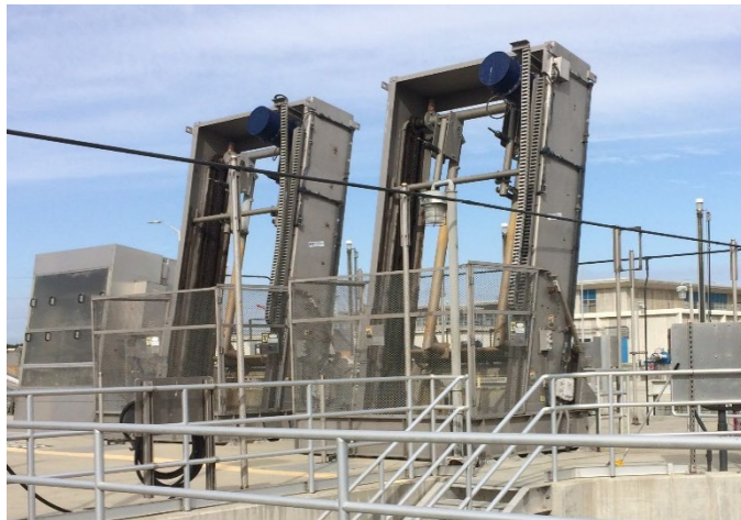
Headworks #1 Bar Screens
