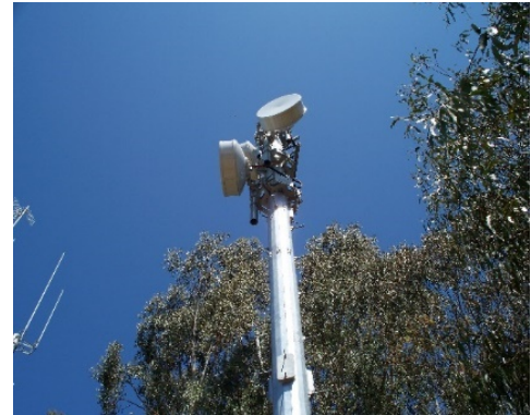
ECOMM Antennae at Eagle Rock
