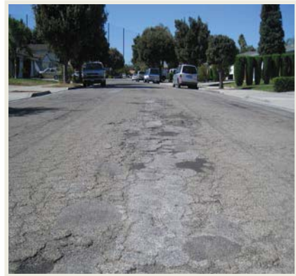
Cheswick Drive – “Poor” Pavement Condition
