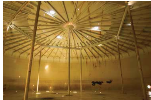
Interior of Nortech Reservoir
