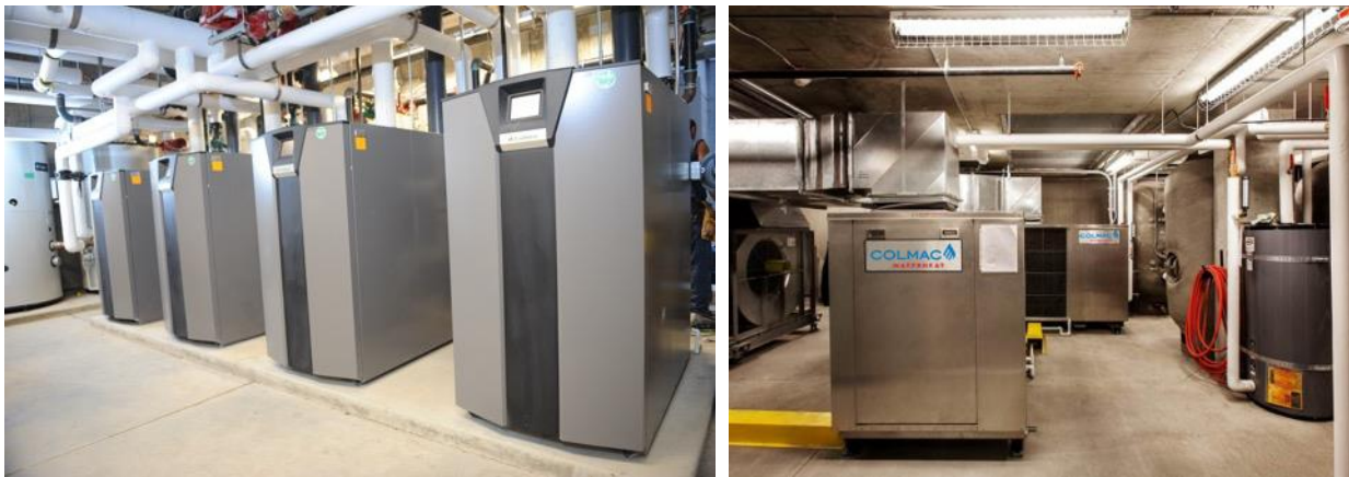
Figure 2: Central gas water heating system (left) and central heat pump water heating system (right).
