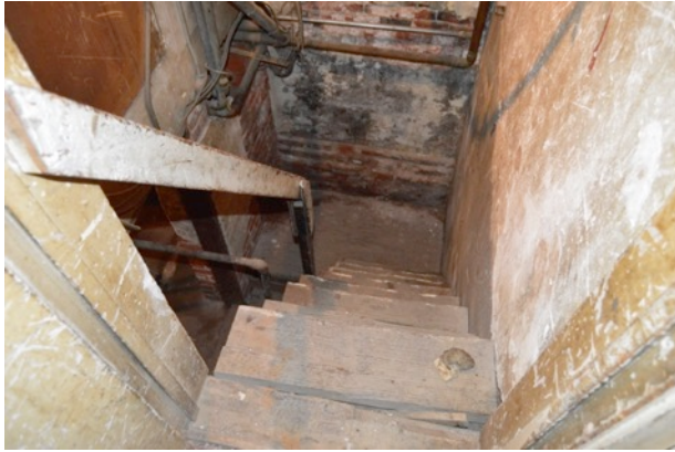
Figure 16. Wood staircase leading to basement at rear of first story, looking east.
