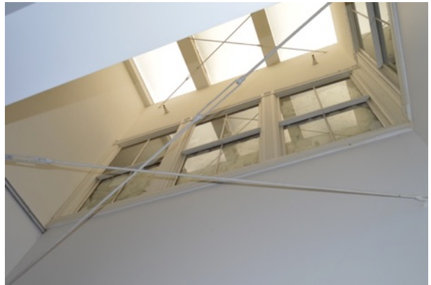
Figure 31. Lightwell and two-over-two wood-sash windows at third story, viewed from second story, looking north.
