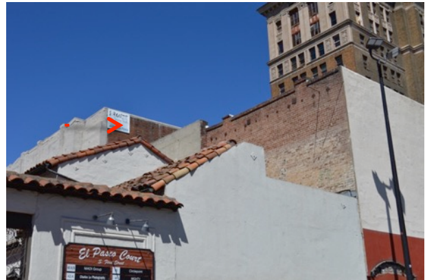
Figure 15. View of a portion of the rear elevation from parking lot along east of subject property, looking northwest.
