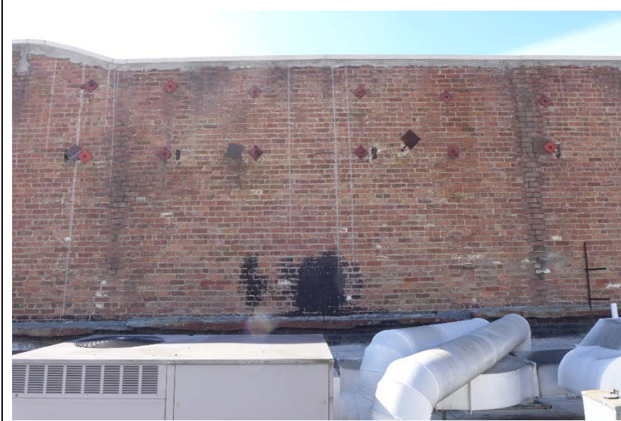
32. Reference photograph. The middle section of the west wall. No major cracks were visible. There were various eras of mortar repairs, but all joints appeared to be sound.
