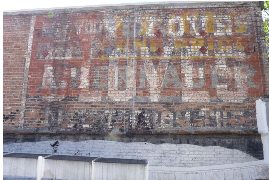
37. It appears that the sign is currently partially covered by roofing and flashing. It is unknown how long it has been that way.
