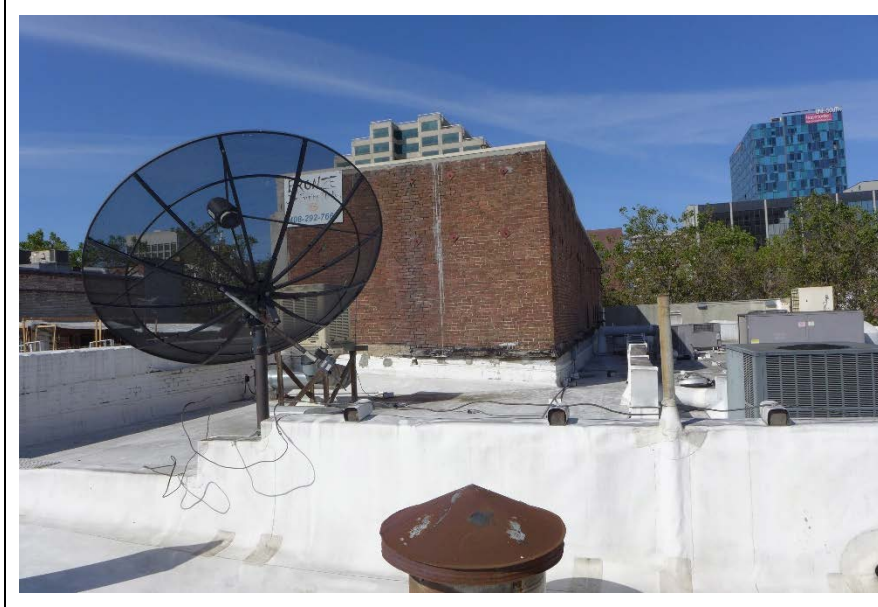
30. Reference photograph. View of the north and west walls of the Knox-Goodrich Building from the roof of the Lido Building.
