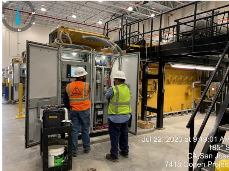
Figure 4 – Testing generators in Building 45
