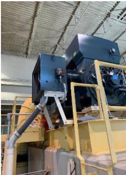
Figure 3 - Building 40 Blower No. 2 Motor
