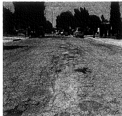
Cheswick Drive – "Poor" Pavement Condition
