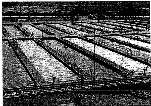
Secondary Aeration Tanks
