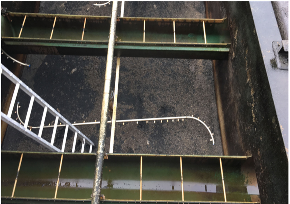
Figure 4: Existing surface wash system which is to be replaced with new air scour system
