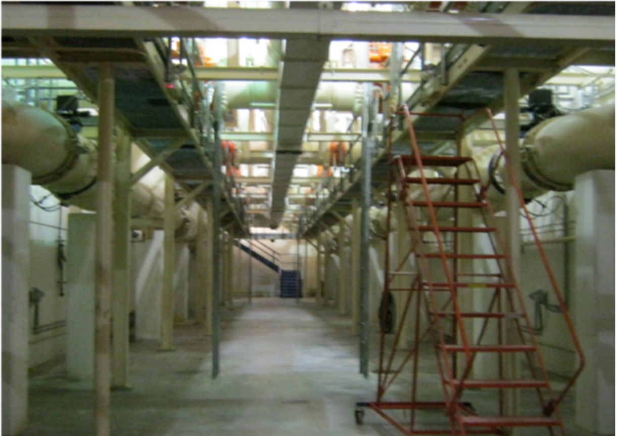
Figure 3: Existing filter galleries which will have 77 valves replaced
