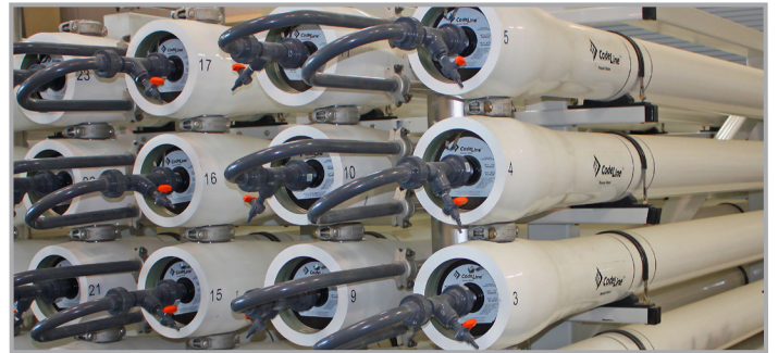
Reverse osmosis vessels at Silicon Valley Advanced Water Purification Center
