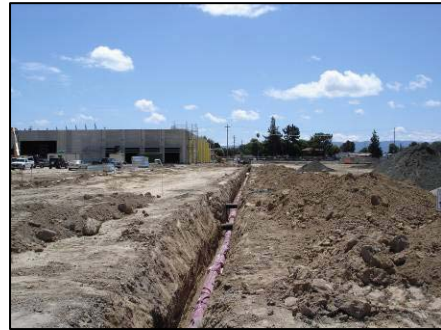
Recycled Water Purple Pipe System
