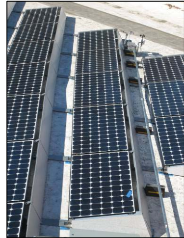
Solar Panels on San José Tech Museum of Innovation
