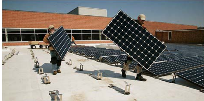
Local Solar Photovoltaic Installation
