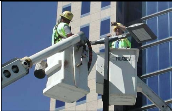
Light Emitting Diode (LED) Streetlights
