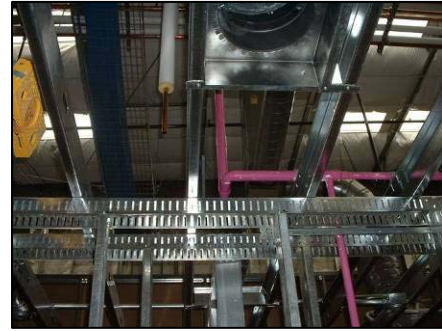
Interior “purple pipe” dual plumbing
