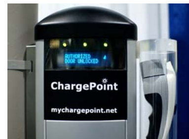
ChargePoint Electric Vehicle Charging Station
