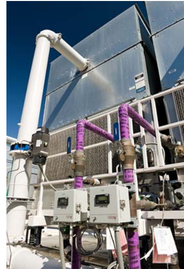
Cooling Tower Using Recycled Water
