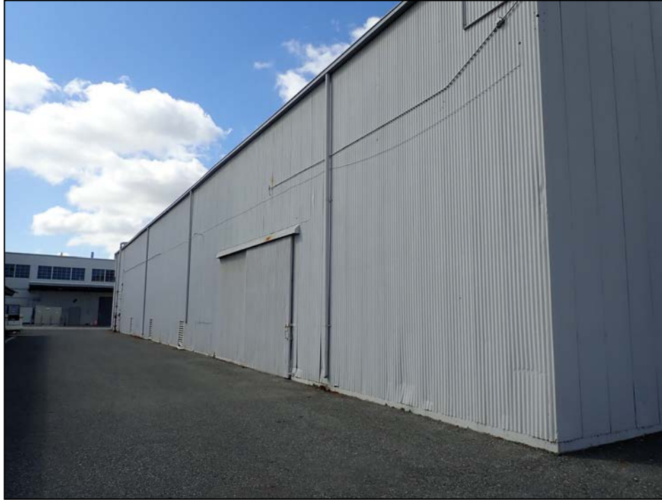
San José Central Service Yard – Building D4. East façade. View to the Southwest. 5/15/20.
