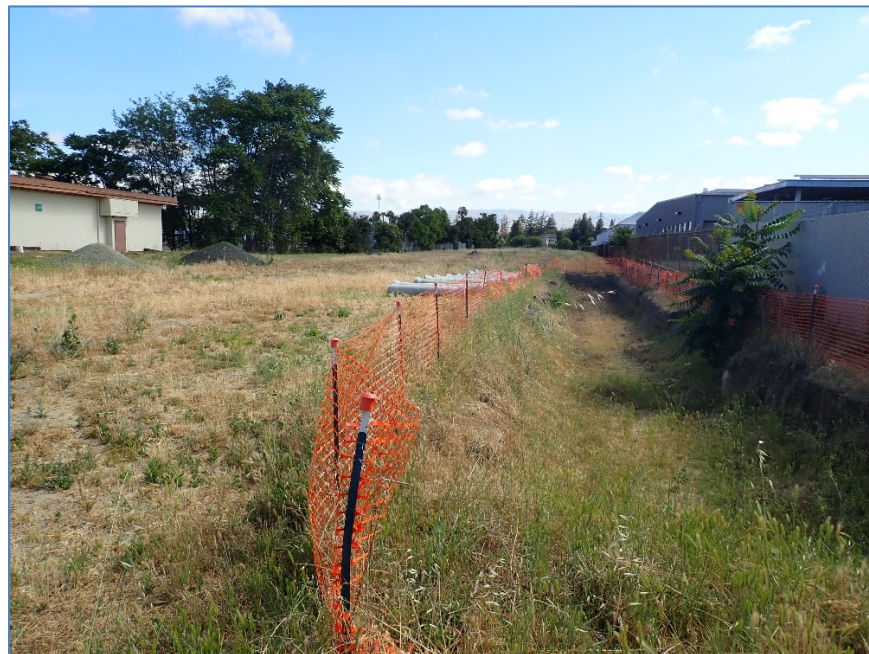
Photo #2: view to NE of southern boundary of Parcel 2 showing utility excavation and staged pipe segments
