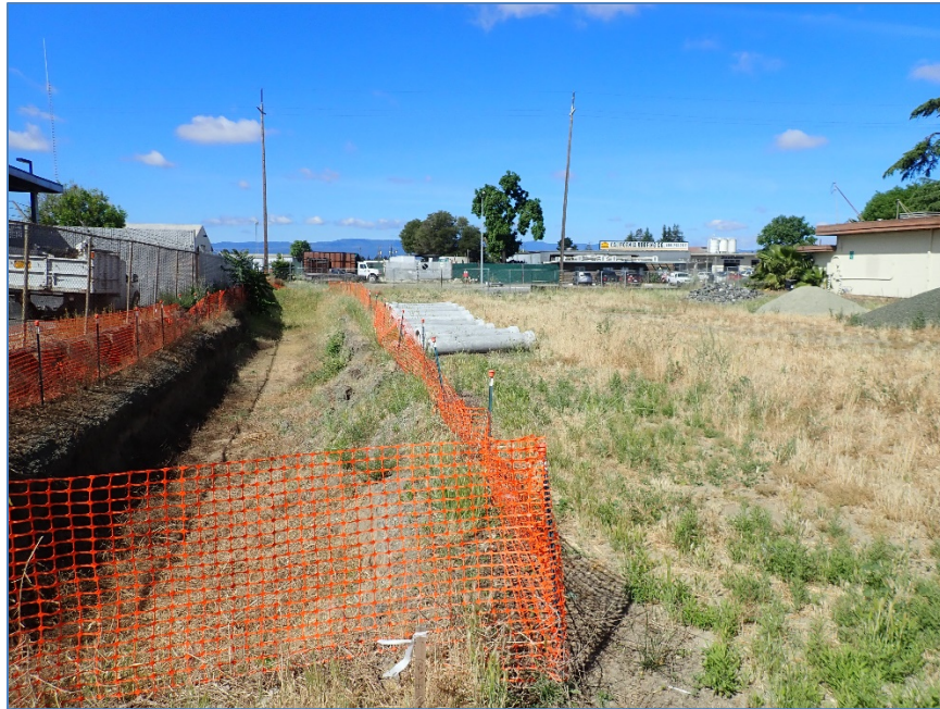
Photo #3: view to SW of southern boundary of Parcel 2 showing utility excavation and staged pipe segments
