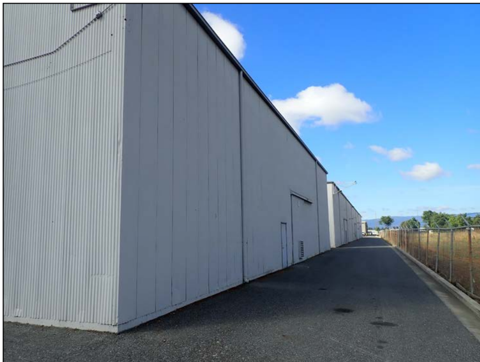
San José Central Service Yard – Building D4. North façade. View to the West. 5/15/20.
