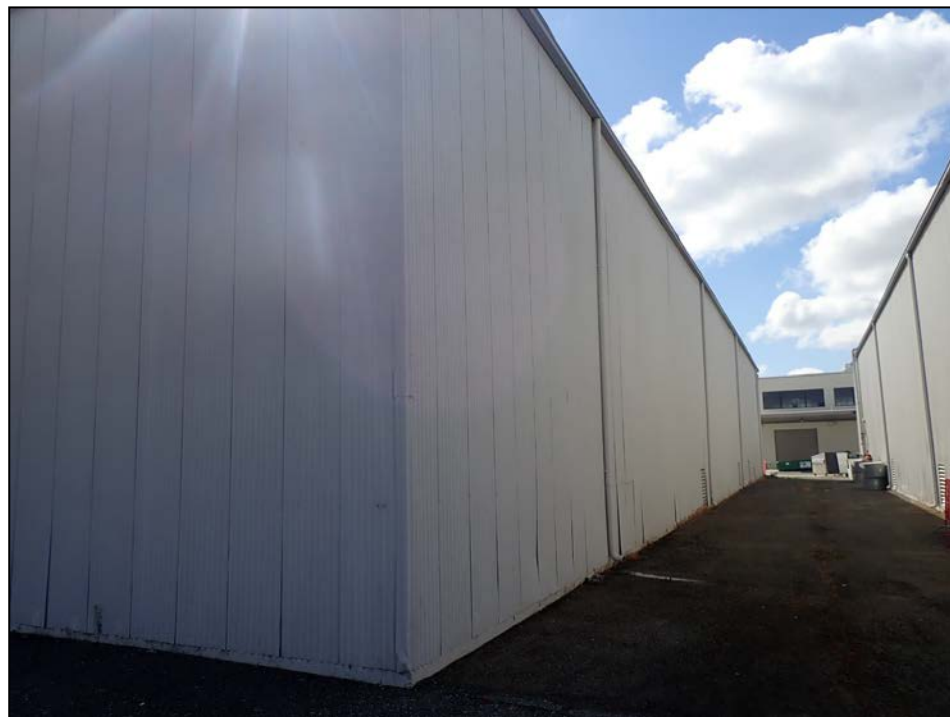
San José Central Service Yard – Building D4. North (partial) and west façades. View to the South. 5/15/20.
