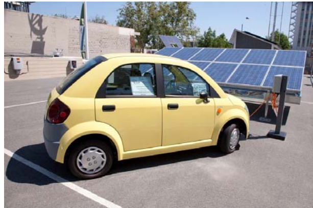
Green Vision Clean Energy Showcase Demonstration of a Solar Powered, Turnkey Electric Charging Station – Collaboration of Breathe California, SunPods, and Aaraya
