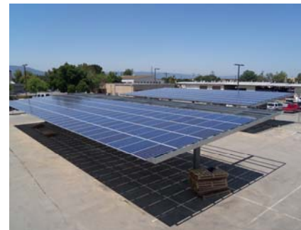
South Service Yard 95 kW Solar System
