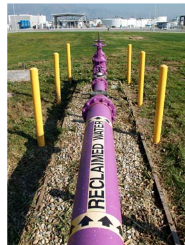
Recycled Water Pipes Photo Credit: Robert Dawson
