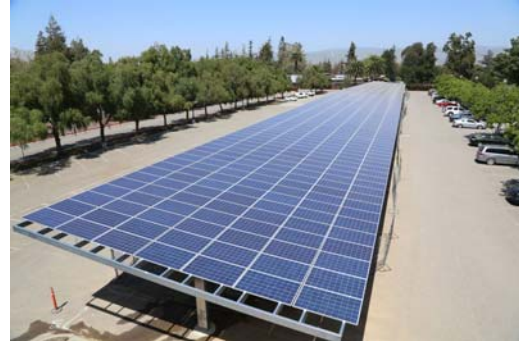
454kW Solar Installation at Happy Hollow Park and Zoo
