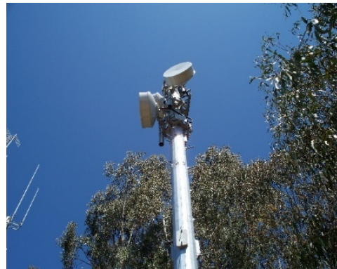
ECOMM Antennae at Eagle Rock
