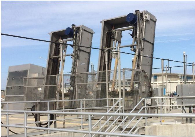
Headworks #1 Bar Screens
