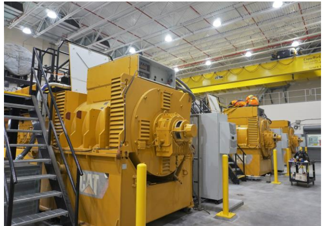
Figure 1 – New Cogeneration Engines
