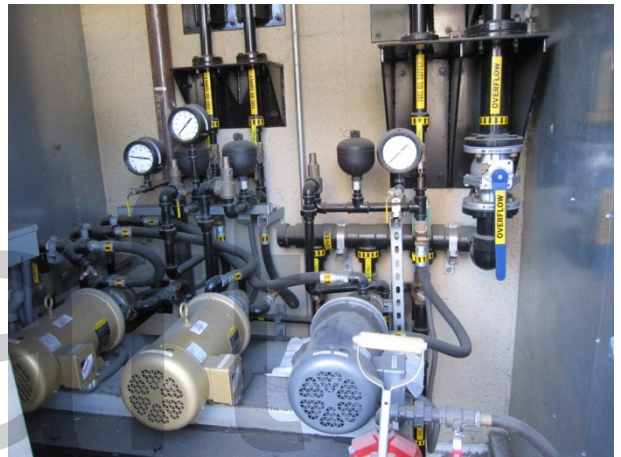
Photograph 10. Fuel pumps within enclosure.
