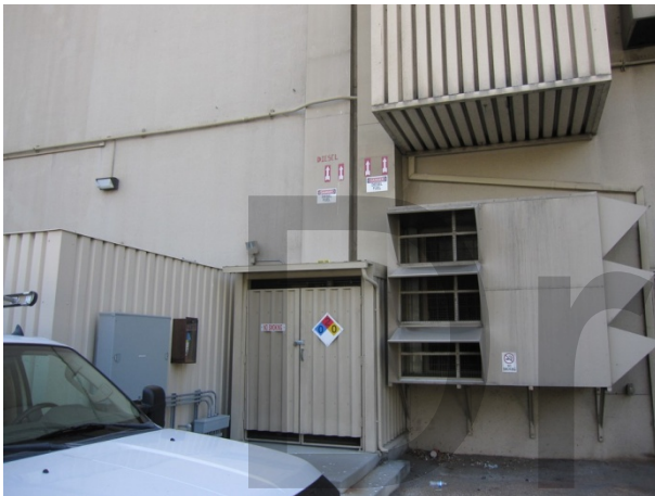
Photograph 9. Current fuel pump enclosure and wall-mounted diesel fuel supply piping.
