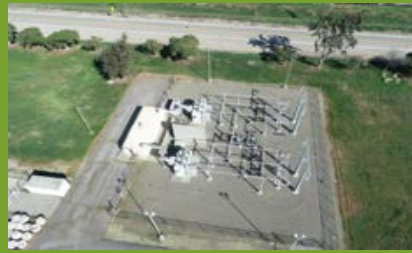
Aerial view of the current Switchgear M4
