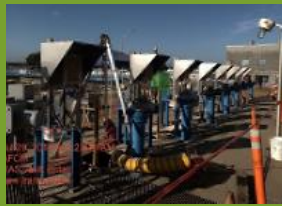
Current RWF control equipment.
