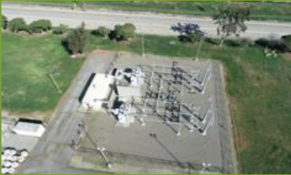
Aerial view of the current Switchgear M4
