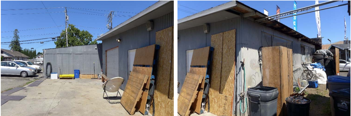
Figures 12 and 13. Southern shed roof addition – east façade (left), and rear shed roof addition – east façade (right).
