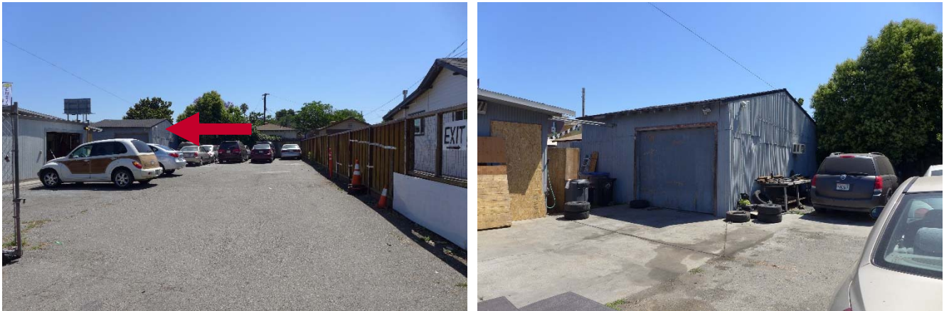
Figures 14 and 15. Rear garage structure identified by red arrow (left) and west and south façades of rear garage (right).
