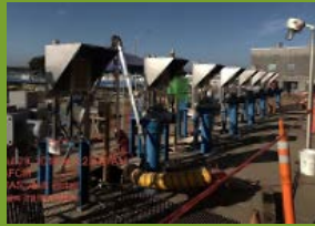
Current RWF control equipment.
