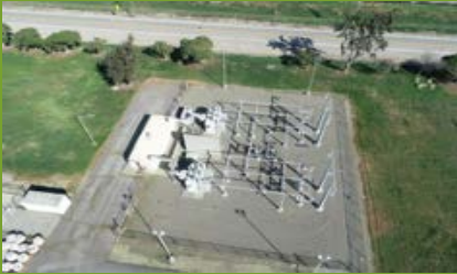
Aerial view of the current Switchgear M4.
