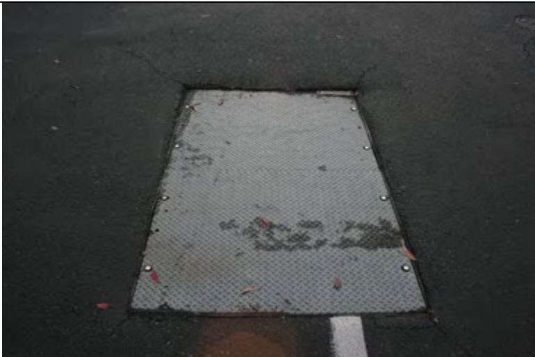
View of on-site utility-owned electrical vault
