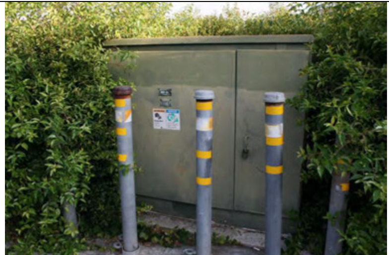
View of on-site utility-owned electrical transformer
