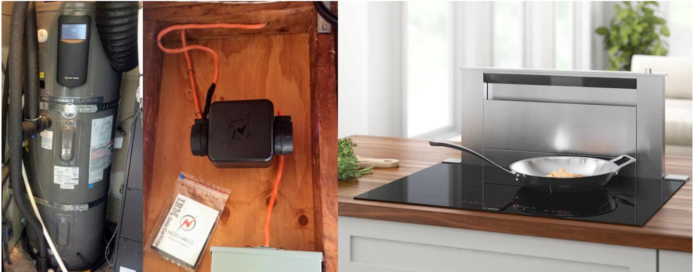
Figure 26: At the Schmidt’s home, the Bosch electric induction stovetop 68 is shared on the same circuit as the Rheem heat pump water heater 69 using the NeoCharge (middle) (Images courtesy of Steve and Lisa Schmidt).
