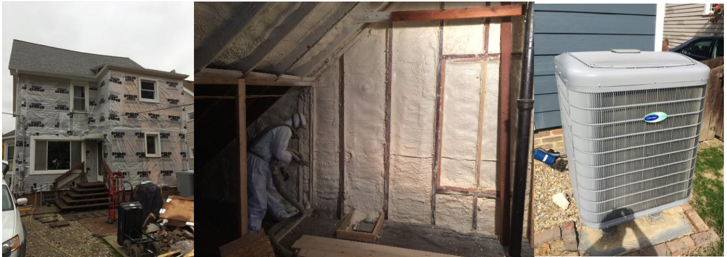
Figure 32: Jon and Kelly's retrofit snap shots, new siding (left), adding insulation, and their Carrier Greenspeed heat pump. 79
