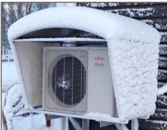
Figure 39: Fujitsu heat pump in the snow. 86
