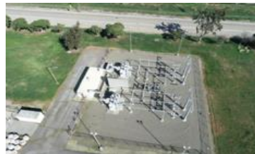
Aerial view of the current Switchgear M4.
