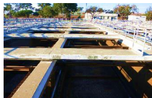
West Primary Clarifiers
