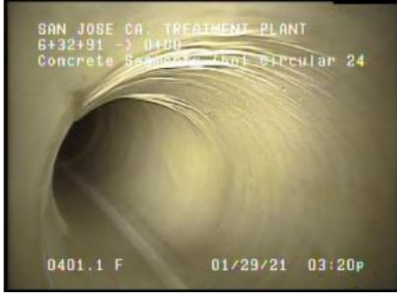
Nitrification Clarifiers Rehabilitation – Phase 1 Project: before (top) and after (bottom) CIPP lining of the 24-inch Nitrification Clarifier RAS lines.
