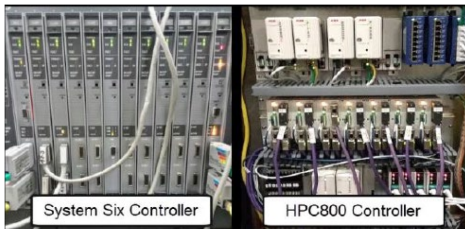
FIGURE 31 THE DCS IS BEING UPGRADED FROM SYSTEM SIX (LEFT) TO NEW HARMONY (RIGHT) CONTROLLERS
