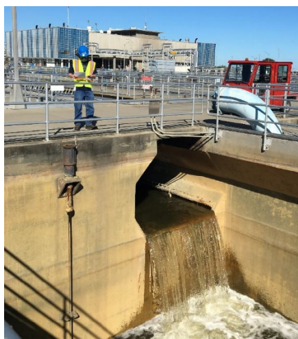
FIGURE 29 A WORKER COLLECTING READINGS AS PART OF THE ONGOING ADVANCED FACILITY CONTROL AND METER REPLACEMENT PROJECT
