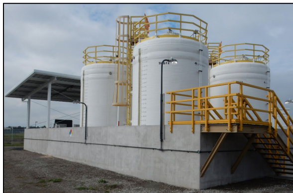
FIGURE 17 IRON SALT FEED STATION
