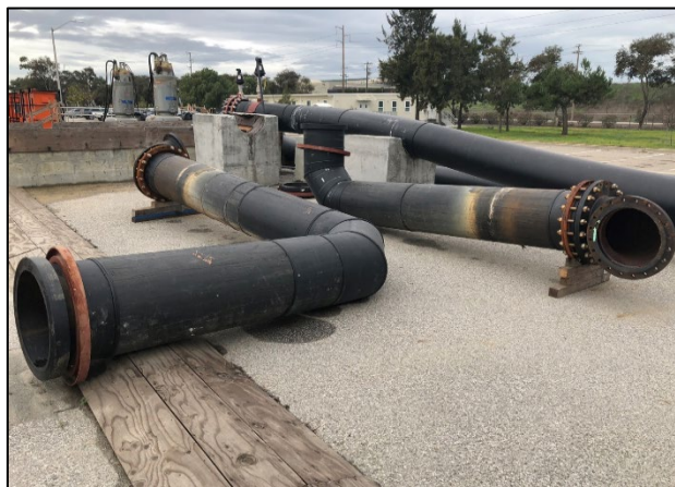
FIGURE 21 SECTIONS OF 36-INCH HDPE PIPE, USED AS A TEMPORARY PIPING SYSTEM IN 2018 THAT WILL BE USED AGAIN FOR THE SES REHABILITATION PROJECT
