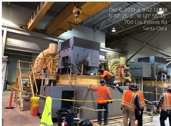
FIGURE 16 BLOWER IMPROVEMENTS PROJECT PREPARING TO INSTALL A NEW ELECTRIC MOTOR TO IMPROVE THE AERATION SYSTEMS’ RELIABILITY
