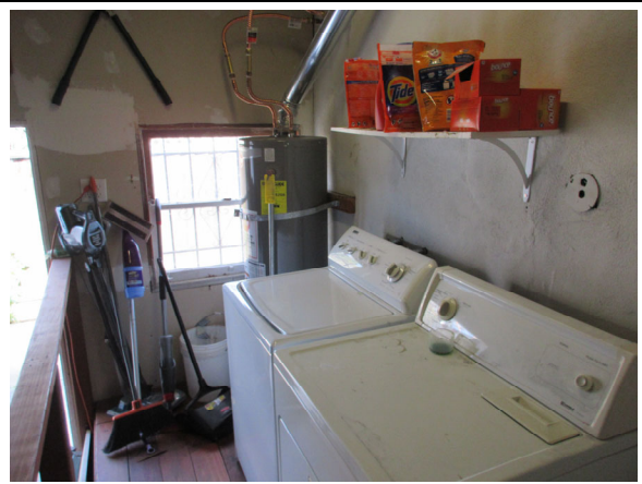
Photo 14: Water heater located in the garage located 383 South Baywood Avenue.
