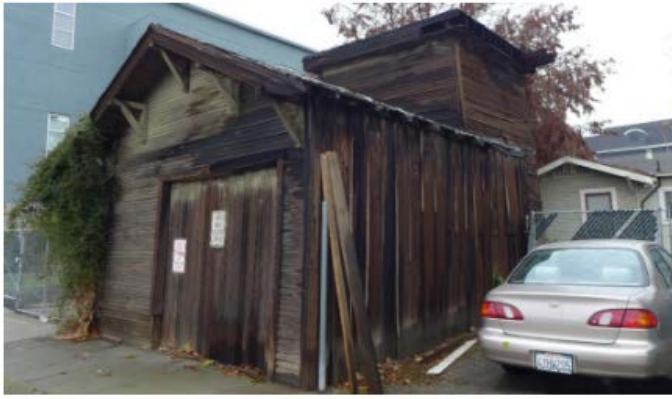
Figure 17. The front (west) and south façades of the tankhouse and the attached garage.
