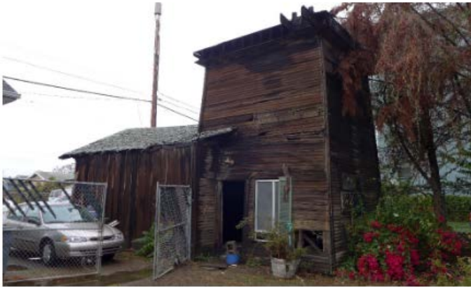
Figure 18. The south and rear façades of the tankhouse and the attached garage.
