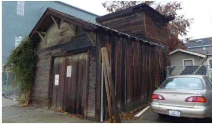
Figure 17. The front (west) and south façades of the tankhouse and the attached garage.
