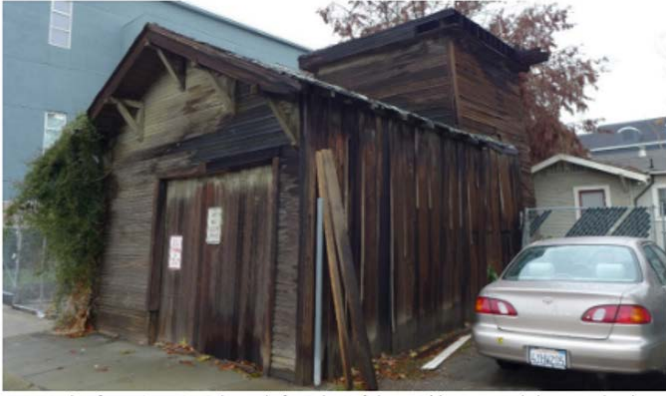
Figure 17. The front (west) and south façades of the tankhouse and the attached garage.
