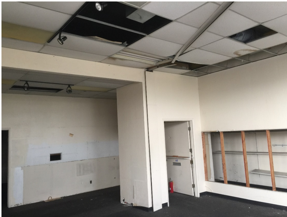
4 – View of the interior of the vacant commercial unit in the eastern portion of the building on the Site. Looking southwest from the northeast corner of the unit.
