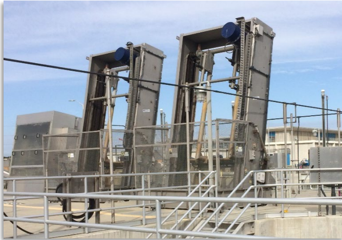
Headworks #1 Bar Screens
