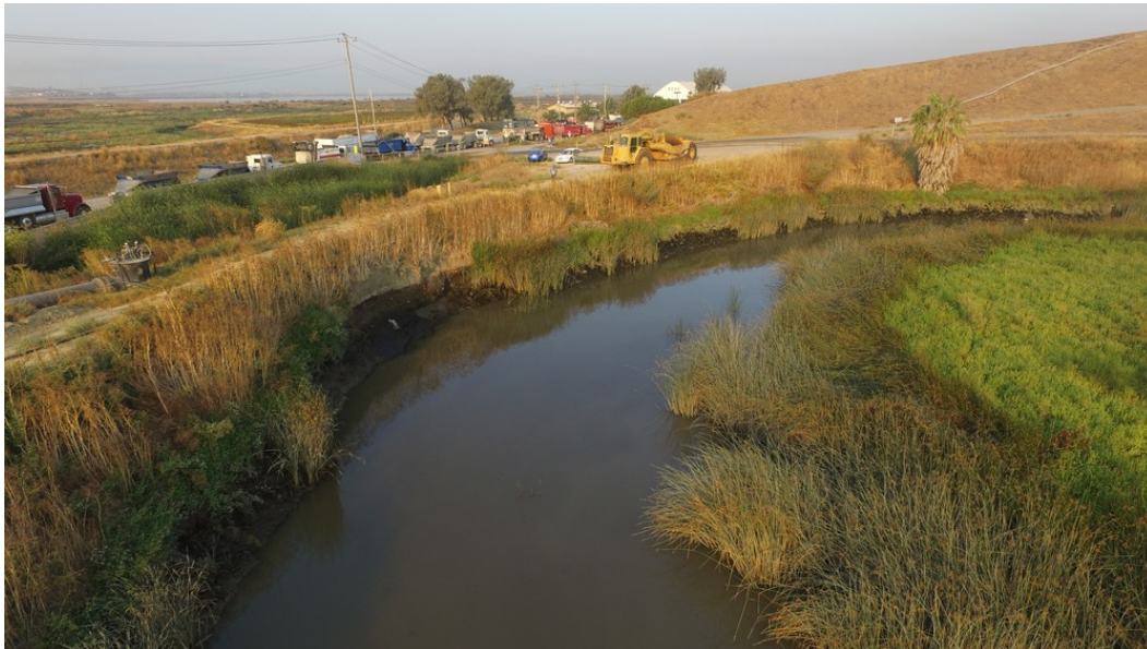
Photo 1: Aerial view of erosion area looking south
