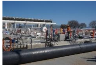
Operational testing at the DAFT.
