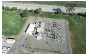
Aerial view of the current Switchgear M4.
