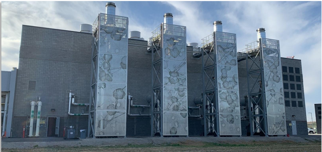
New Cogeneration Engine Building
