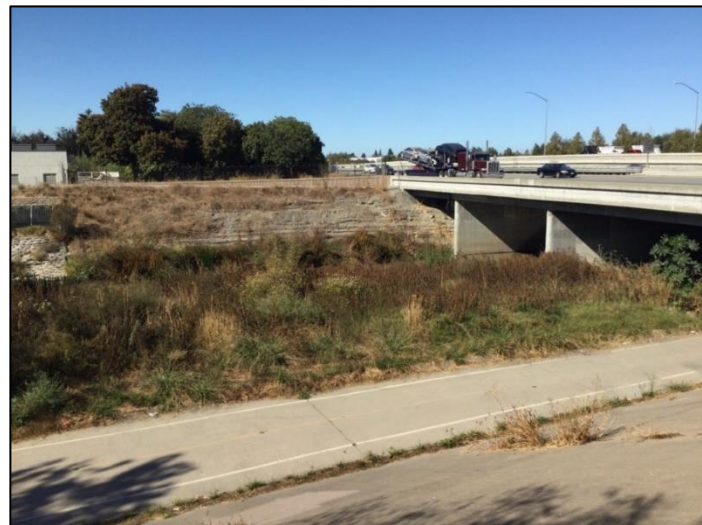
Photo 6. Looking west down to the Guadalupe River Trail at the bottom of a concrete-paved slope, from the Valley Water gravel service road, west of the south project site. Hwy 101 is shown crossing over the Guadalupe River.
