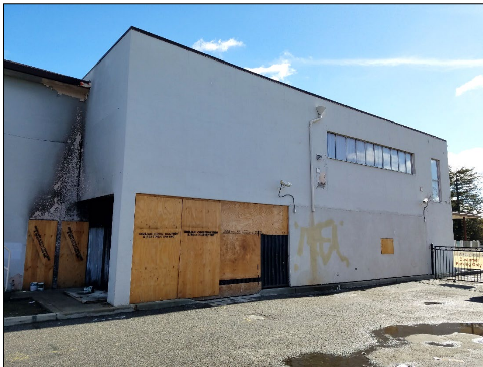
Photograph 3. West wall of concrete quadrant and infilled bay, camera facing east, February 12, 2021.
