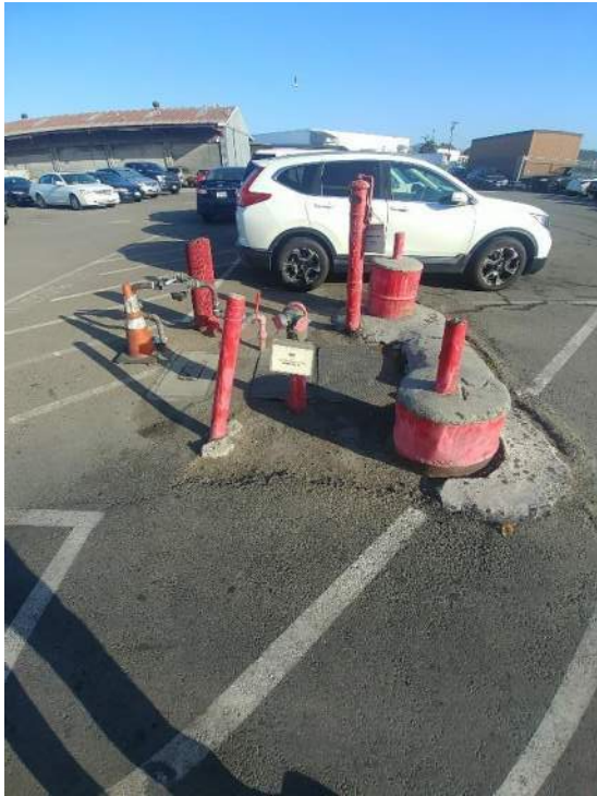
Photograph 27. Fire suppression water supply to the Site. Located in the Recycling Specialists parking lot, near Old Bayshore Highway.
