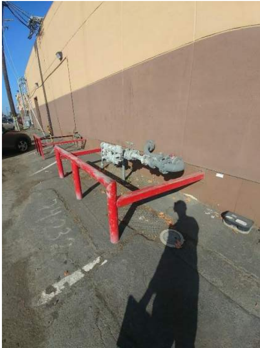
Photograph 5. PGE gas supply on the south side of the Smithfield facility.
