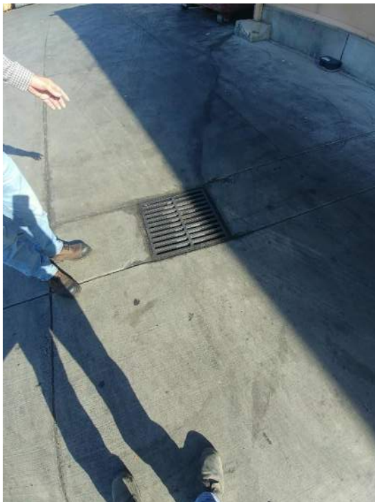
Photograph 8. The Smithfield facility also has storm water catch basins that drain directly to the municipal storm sewer. This drain is located in the driveway on the west side of the packing operations.
