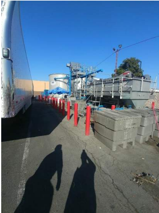
Photograph 9. Water treatment system located in the northern portion of the Smithfield facility. The system has a grease removal component, and a pH balancing portion. Discharge pH is regulated by titration with proprietary solution containing sodium hydroxide.
