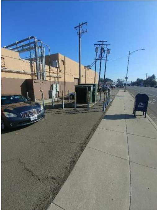
Photograph 3. Pad-mounted and pole-mounted, PGE owned transformers.
