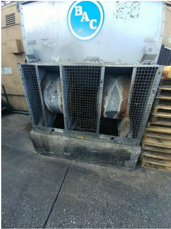
Photograph 13. Air-conditioner at the Smithfield facility. The other A/C units are roof-mounted. This unit is mounted on an 8-inch pad that appears free of staining.
