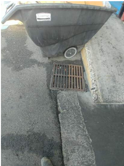
Photograph 6. Water catch-basin on the north side of Smithfield packing operations. This catch-basin feeds a grease-trap and water treatment system.
