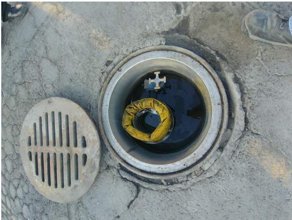
Photograph 16. Storm water catch basin outfitted with a silt filter. There are four storm water catch basins on this facility; three have the silt filter.
