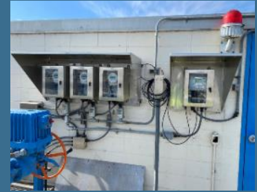
New flow meter transmitters with weather protective enclosures at Secondary RAS Pump Station.
