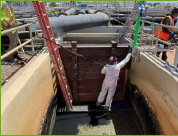
Stop logs installed at the North Settled Sewage Vault.
