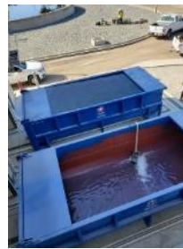
Pre-operational testing at the Sludge Screening Building.
