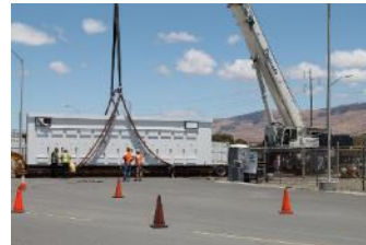
Arrival of the new Power Control Room
