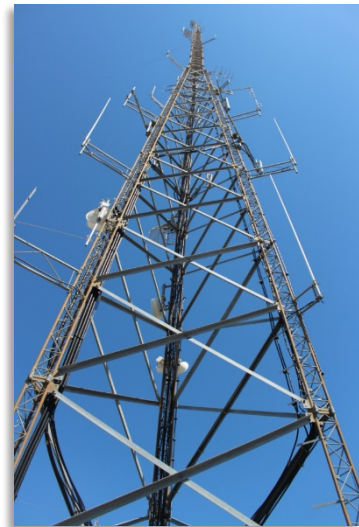
Transmitter Antennae at Coyote Peak
