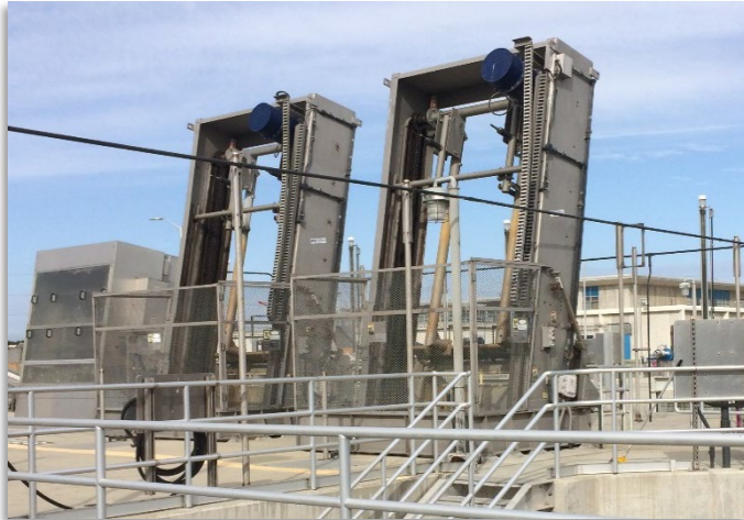
Headworks #1 Bar Screens
