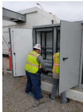
Contractors testing in the new battery enclosure.
