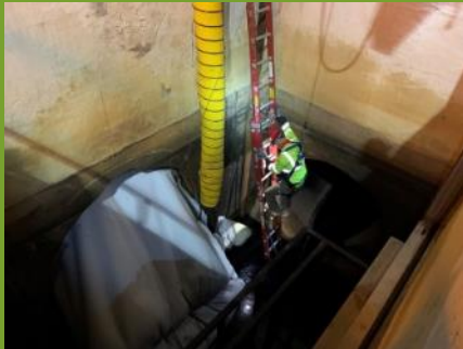
Contractor at the end of the cured-in-place pipe liner at the 96-inch primary effluent junction box.
