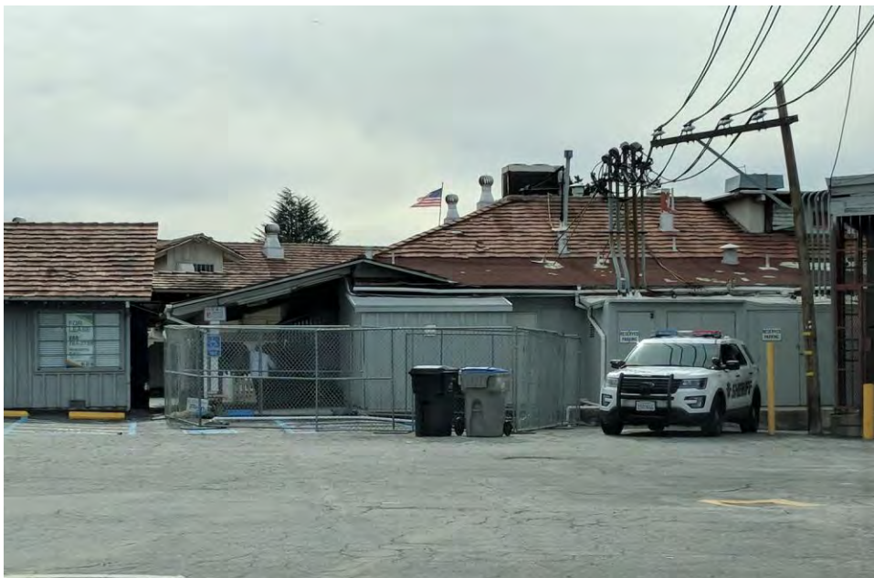
Rear of Breezeway Between Central Wing and Southern Shops. Viewed facing Southwest. July 2018.
