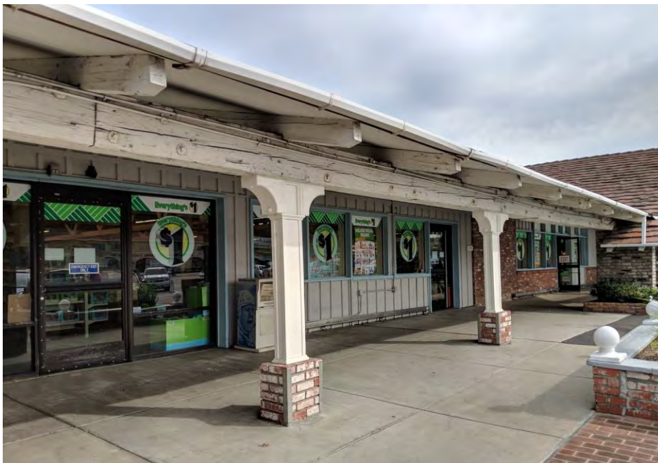
North Corridor of Central Wing. Viewed facing Southeast toward anchor store. July 2018.
