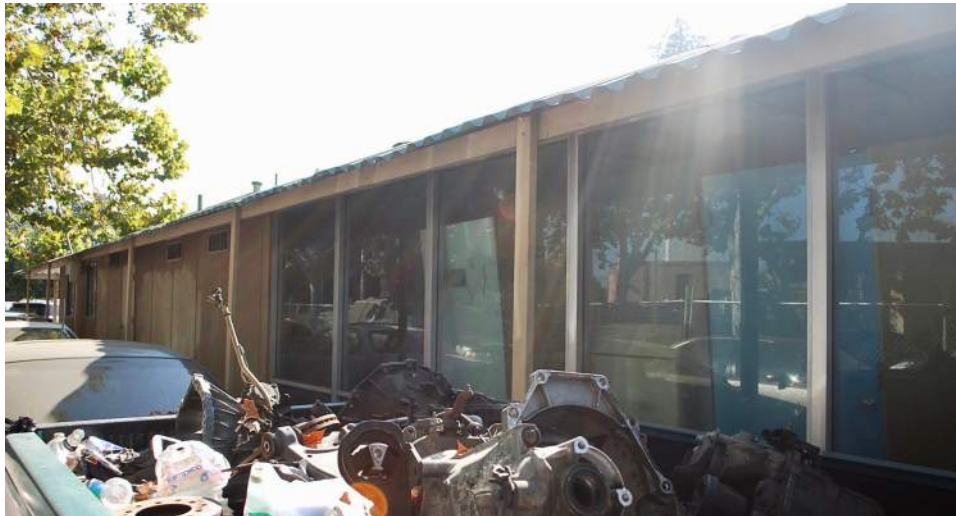
Three views of the north wall of the building. The aluminum windows are a wrap-around from the Bascom Avenue front; plywood siding is to the rear.
