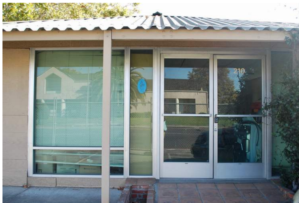
Aluminum window, sidelight, and paired doors on the Bascom Avenue front of #210
